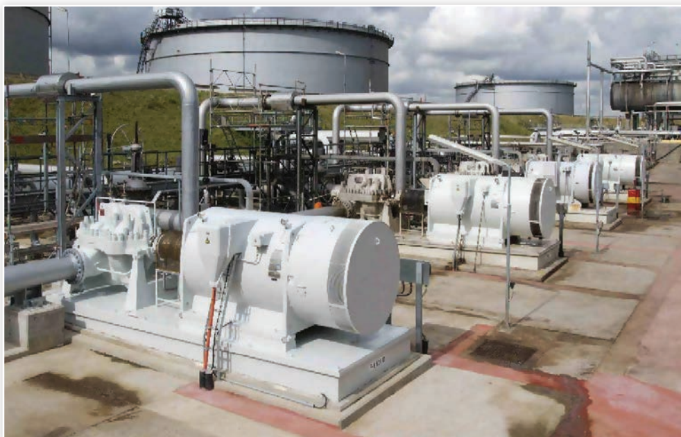
Drives for crude oil pumps, Ex db (ec) IIB T4, 1.500 kW, 10 kV, 4-pole
